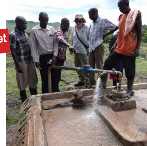
KKI was able to provide funding to fix an existing bore by supplying new solar panels, a new pump and pipework. Over 3,000 people benefit from clean water being available as well as the local school.
